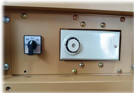
Unit Mounted Controls
